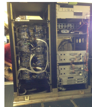
Radar Transceiver and Processor Rack (2 out of 4 shown)
